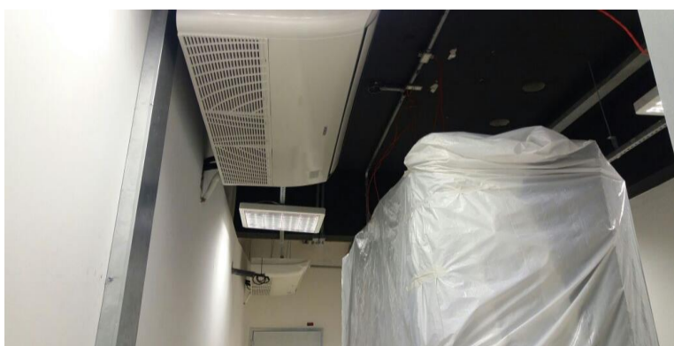
EQUIPAMENTOS AR CONDICIONADO - CPD/ AIR CONDITIONING EQUIPMENTS - IT ROOM
