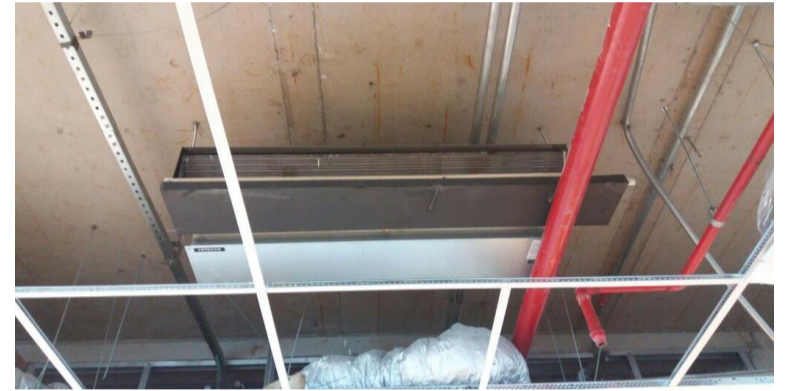
EQUIPAMENTOS AR CONDICIONADO - STAFF/ AIR CONDITIONING EQUIPMENTS - STAFF
